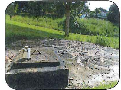
Keep septic tanks sealed.
